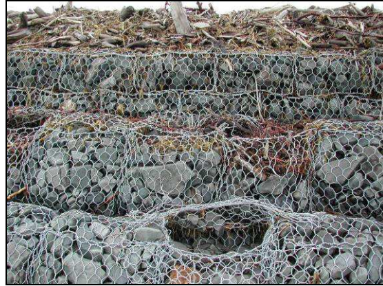
Typical Gabion Cell Rupture
