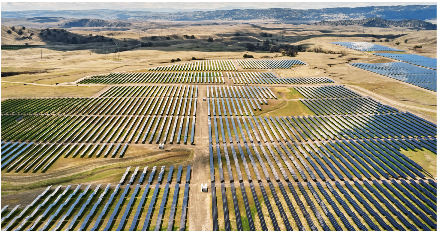
Apple helped create a new utility-scale battery storage project that supports the 130-megawatt California Flats solar farm, which provides renewable energy for our California facilities.
