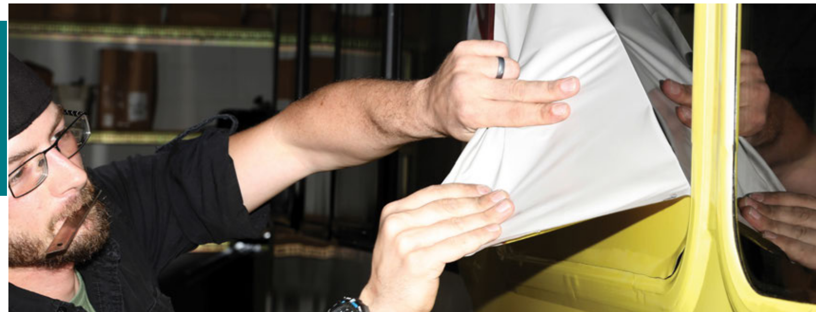
Andrew Reininger from AdVenture Installation puts the new exterior on the CRE bus.
