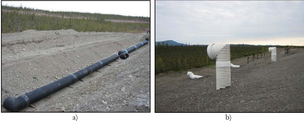
Figure 11: a) Longitudinal culverts placed in trench with some heat shrinking complete (blue joints) and prior to heat shrinking and backfill. b) Finished longitudinal culverts showing inlets (horizontal pipes) and outlets (upright pipes).
