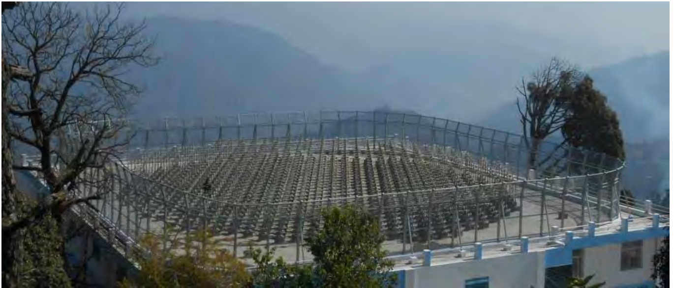
Fig. 2: Recently installed a clutter fence along the periphery of the ST Radar antenna array on the rooftop of the building.
