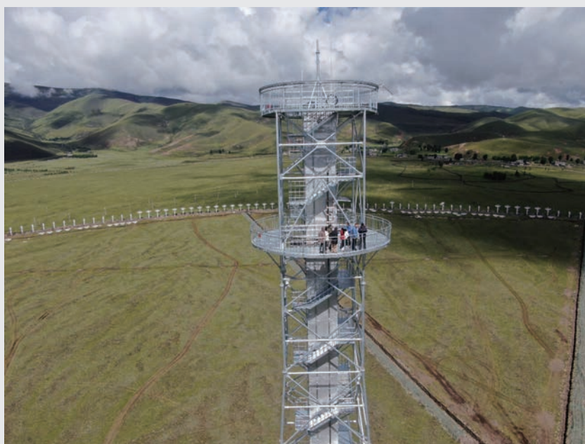
Daocheng Solar Radio Telescope (DSRT) of the Meridian Project (II) is under construction
