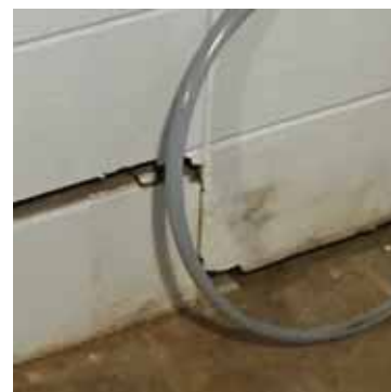
Block Wall Failure
