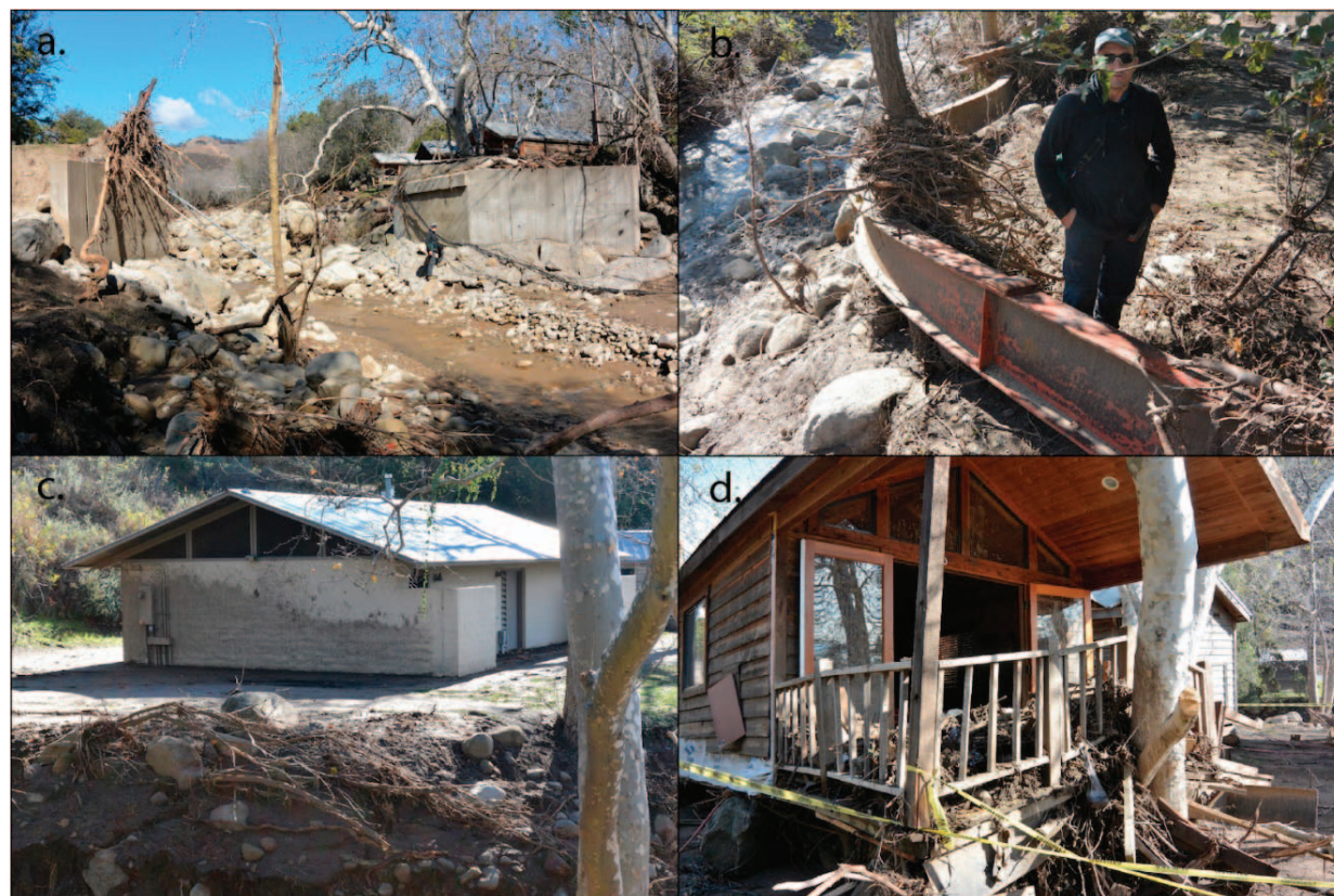
Figure 10. (a) Damage to the Mid-Canyon Bridge, supported on both sides of the creek by concrete abutments. (b) Twisted metal I-beams that supported the Mid-Canyon Bridge prior to the debris flow event. (c) Structure on the flood plain marked on its up-stream side by mud patinas to a height of up to 2.5 m. (d) Damaged cabins at the El Capitan Canyon Resort.
