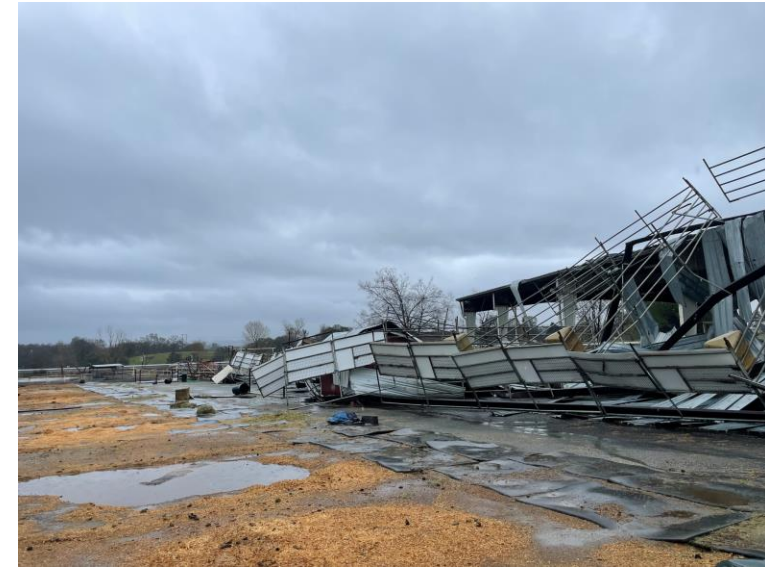
Tornado damage to a 17-stall horse barn kcranews Twitter
