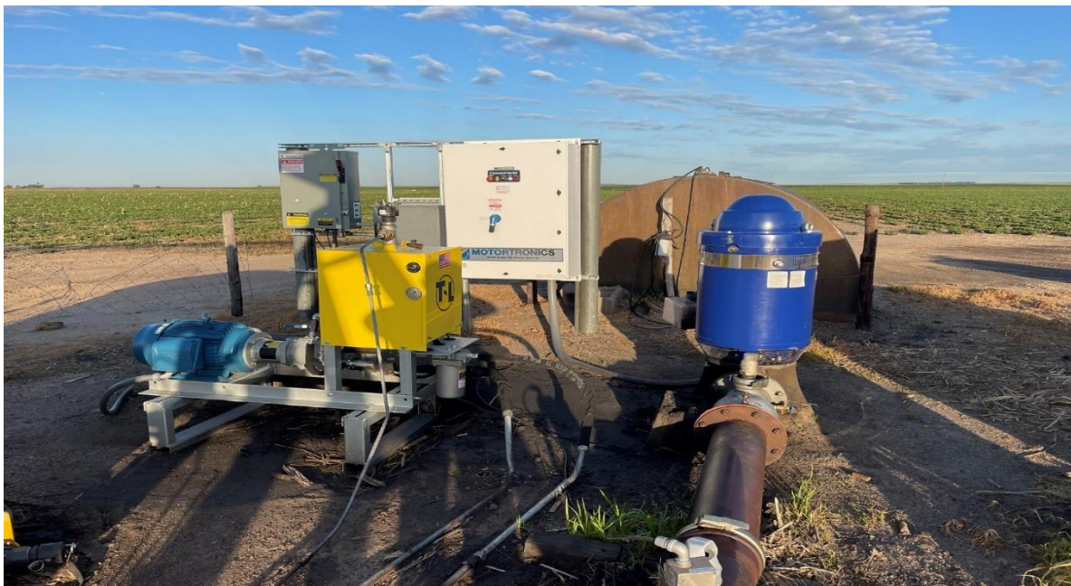
New electric motor and related equipment replacing a diesel engine at an irrigation well in Lincoln County, partially funded by the 2022 Nebraska Clean Diesel Rebate Program. Photo courtesy of the owner.
