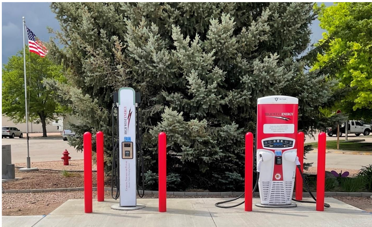
Level 2 (left) and DC fast charger installed at the High West Energy Service Center in Potter (2 miles from Interstate 80 in western Nebraska) and partially funded through the Nebraska Electric Vehicle Charging Rebate Program. Photo courtesy of High West Energy.
