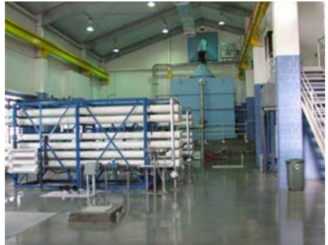
Reverse Osmosis treatment plant to remove nitrate, Seward County.
