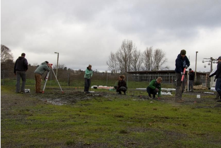
Figure 12: Toby Bloom, UW Construction Management student, determining the height of each corner to set a level foundation for the hoop house.
