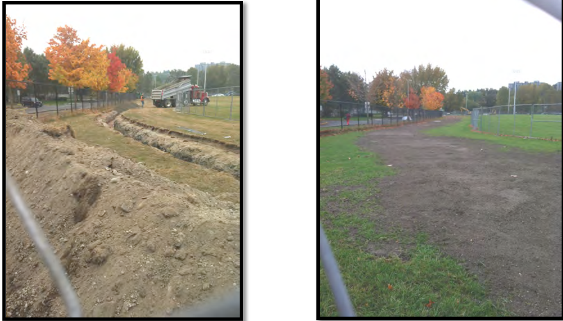
Figure 2: Soil disturbed during construction of an irrigation pipe for the Intramural Fields at the University of Washington. Soil was mechanically excavated one day and stockpiled during the pipe construction (photo on left). The soil was then replaced two days later (photo on right). The area was then hydro-seeded making the large amount of soil excavation and replacement almost invisible.
