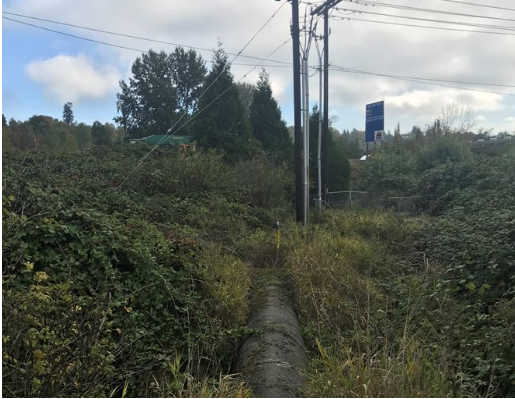
Figure 40: Photograph of the Norfolk Pumpstation, including water-transport infrastructure.
