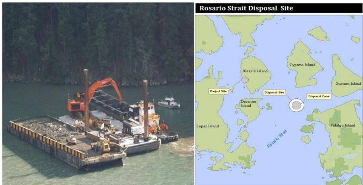
Figures 4 and 5. Sediment excavation (left) and location of dispersal site (right). Source: SFEG.
