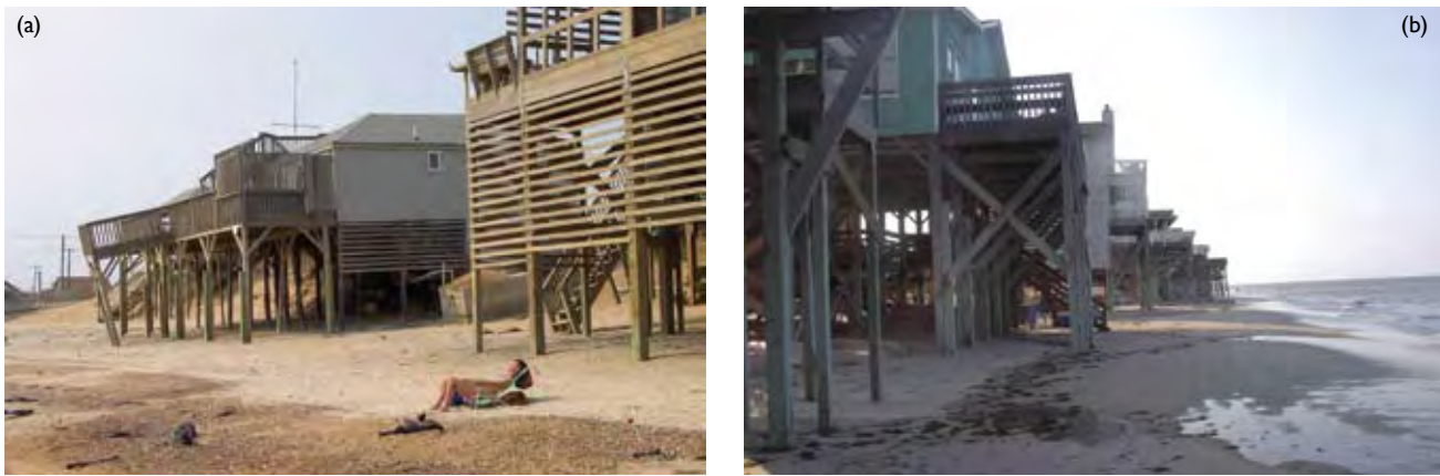
Figure 6.9 The adverse impacts of retreat on safety and aesthetic appeal of recreational beaches. (a) Exposed septic tank and condemned houses at Kitty Hawk, North Carolina (June 2002); (b) Beach unavailable for recreation where homes were built to withstand shore erosion and storms, at Nags Head, North Carolina (June 2007) [Photo source: ©James G. Titus, used with permission].
