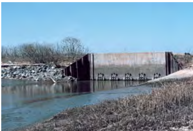
Figure 6.5 The tide gate at the mouth of Army Creek on the Delaware side of the Delaware River. The tide gate drains flood and rain water out of the creek to prevent flooding. The five circular mechanisms on the gate open and close to control water flow [Photo source: courtesy NOAA Photo Library].
