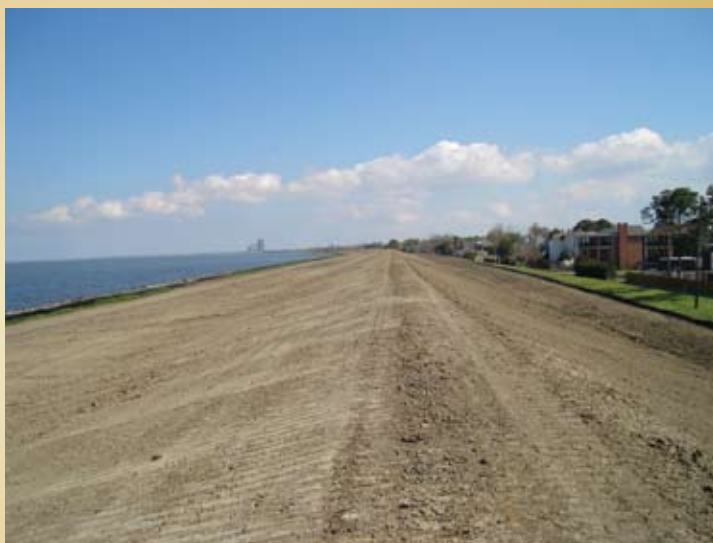
Recent upgrades that raised the height of this earthen levee increased protection against storm surge in the New Orleans area.
