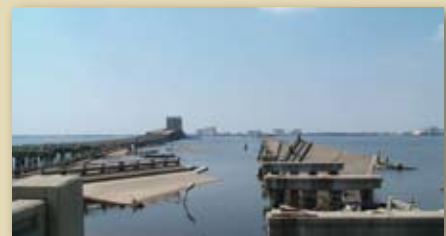
Hurricane Katrina damage to bridge
