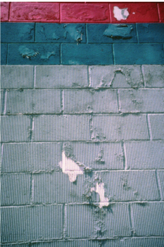
Figure 1-6 Blistering paint on split face concrete block. Wind-driven rain is the source of moisture contributing to the damage. Water wicks into the concrete masonry unit (CMU) through pin holes in the paint. The sun drives water vapor through the CMU. The assembly cannot dry to the interior because low-vapor-permeability foam board, taped at the joints, insulates the interior surface of the wall. The wall remains saturated throughout the spring, summer and fall. The same paint on areas of the wall sheltered from sun and rain shows no damage.
