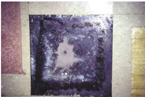
Figure 1-13 Tile adhesive that failed to cure because of water in the concrete and high pH. The tile can be removed by hand. The floor is a concrete slab-on-grade. The water visible in the photo evaporates into the room after several minutes. Its source may be liquid water wicking up from the sub-slab fill or water vapor migrating through the slab.
