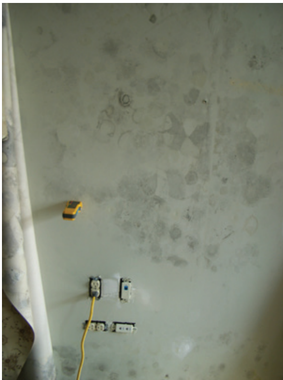
Figure 1-7 Condensation behind vinyl wallpaper in a warm, humid climate. Condensation and mold growth occurs behind the vinyl wallpaper on both exterior and interior walls. Air leaks in the return plenum of the air handler depressurizes the interior and exterior wall cavities. Warm, humid exterior air is drawn from outside through air leaks in a heavy masonry wall.
