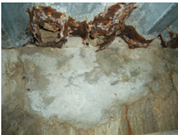
Figure 1-4 Corrosion of galvanized fluted steel floor deck. The floor is at grade level. The source of the water is rainwater seepage.
