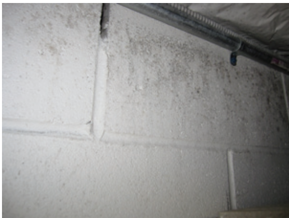
Figure 1-2 Mold growth on painted concrete masonry. The cool masonry wall separates a classroom from an ice rink. Humid air in the classroom provides moisture that condenses on the painted surface of the masonry. That moisture allows mold to grow on the paint film.
