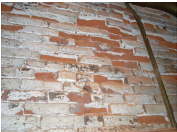
Figure 1-14 Damage to bricks caused by the migration of soluble salt through them. Salts in the brick or mortar dissolve in rainwater that wicks through the brick. The water evaporates in the building's interior, and the salt left behind crystalizes and splits the surface layer off the brick, exposing its interior. This process is called sub-fluorescence.
