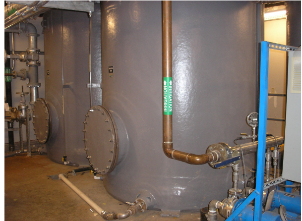
Two 2,500-gallon tanks storing air handler condensate and harvested rainwater for irrigation
