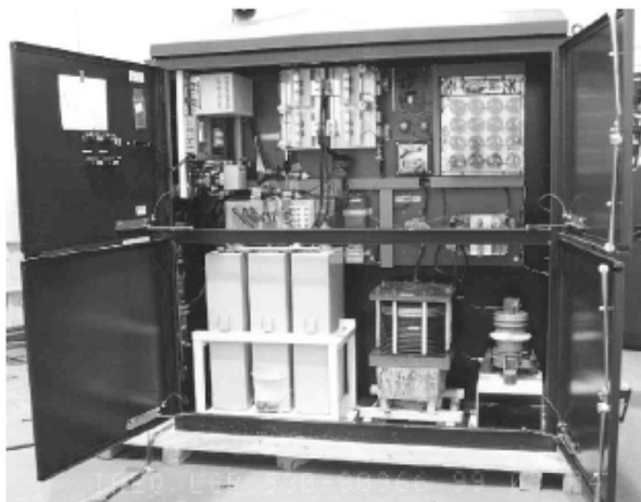
Figure 27: Neutral current blocking device (NCBD) installed in the neutral of a three-phase transformer as a year-long test by Hydro Quebec [7].
