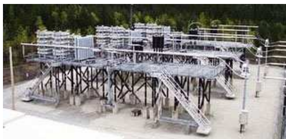
Figure 26: A three-phase series capacitor for a EHV transmission line. Warranted economically under most circumstances, installations like this pay back over many years but would be difficult to mandate only for GIC mitigation.
