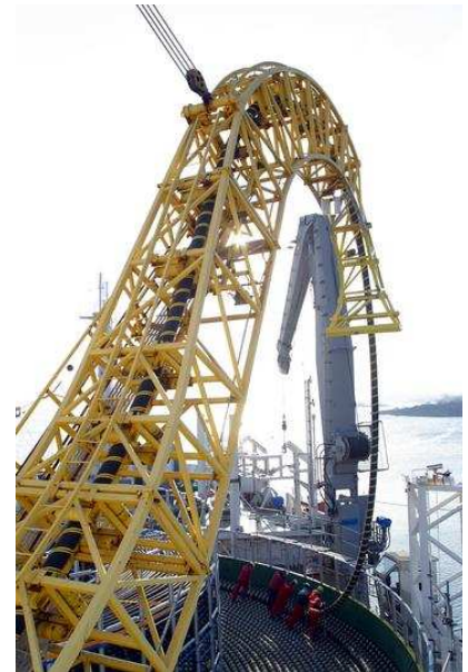
Figure 25.7. Laying a high-voltage DC link between Finland and Estonia. A pair of these cables transmit a power of 350 MW. Photo: ABB.
