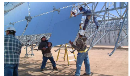
Figure 25.4. Andasol – a “100 MW” solar power station under construction in Spain. Excess thermal energy produced during the day will be stored in liquid salt tanks for up to seven hours, allowing a continuous and stable supply of electric power to the grid. The power station is predicted to produce 350 GWh per year (40 MW). The parabolic troughs occupy 400 hectares, so the power per unit land area will be 10 \text{ W/m}^2 . Upper photo: ABB. Lower photo: IEA SolarPACES.
