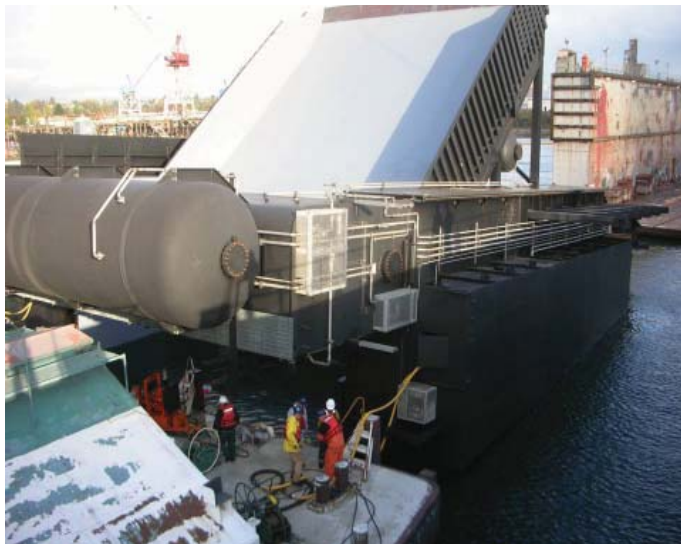
Removable Surface Weir (RSW) for Ice Harbor Dam. Photo: US Army Corps of Engineers.
