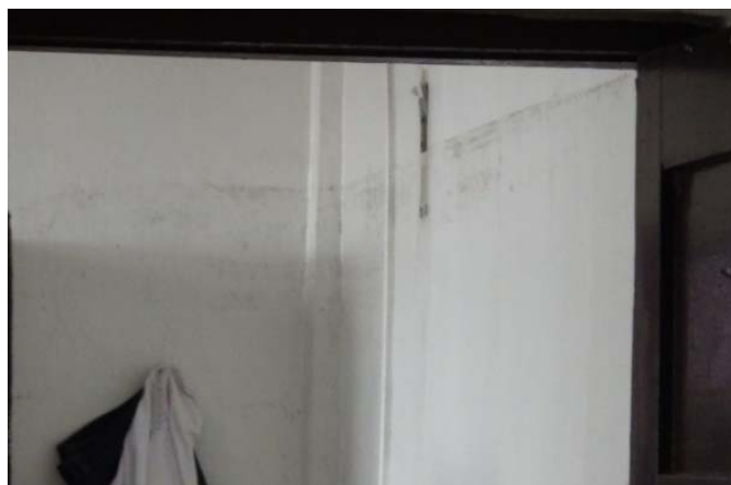
Fig.5-7. Water line inside a building in inland downtown Tacloban.
