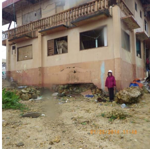
Fig.5-27. Scour up to 1 m deep around foundation in Hernani.
