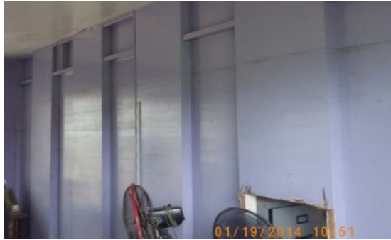
Fig.5-8. Water line inside a building in inland downtown Tacloban.
