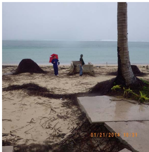
Fig.5-22. Damage near Guiuan PAGASA station. Damaged foundation located 4 m above Mean Sea Level.
