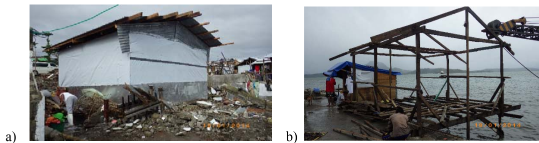
Fig.5-11. a) A house rebuilt with corrugated galvanized iron sheet and wooden studs, b) A house being rebuilt with debris.
