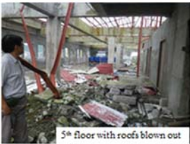
5 th floor with roofs blown out
