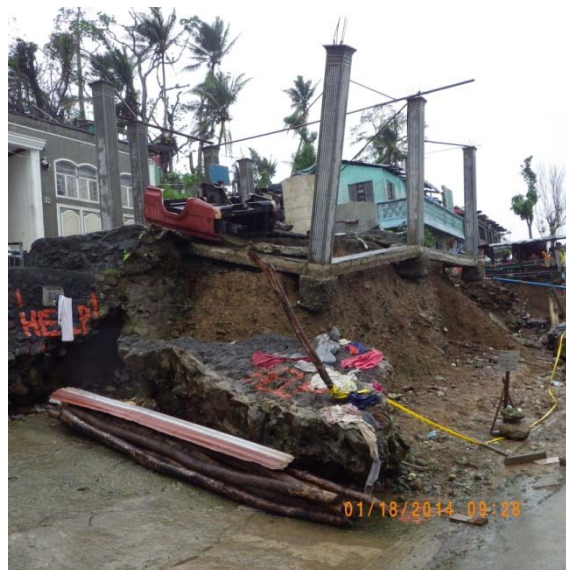
Fig.5-13. Scour of building foundation in coastal downtown Tacloban.
