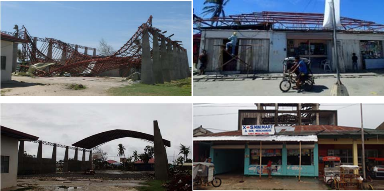
Fig.9-11. Completely damaged buildings in Barangay Kawit, Cebu (before and after repairing) Basketball gymnasium (left) and private concern (Right)
