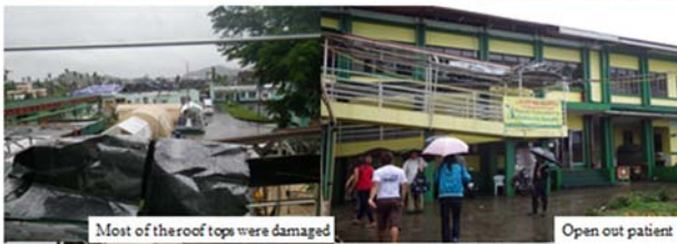
Most of the roof tops were damaged
