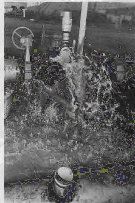
After a hard day in the field, worker takes a makeshift bath in pesticide contaminated water from an irrigation pipe.
