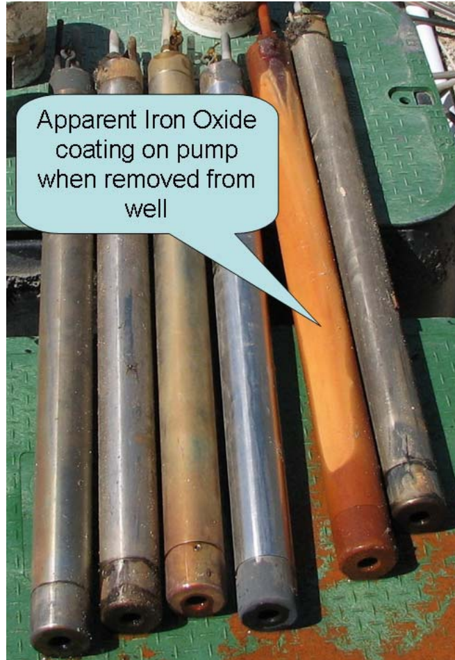
Figure 20. Pumps after approximately 18 months of continuous operation.
