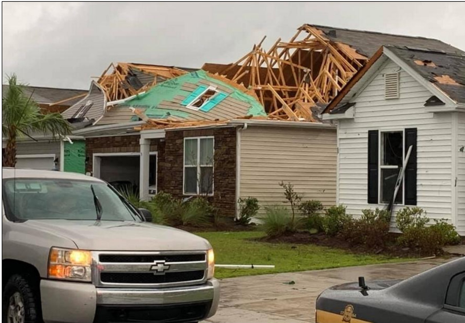
Figure 11. Roof damage to homes in Brunswick County, North Carolina, caused by an EF2 tornado on 5 September 2019. Picture courtesy of Brunswick County Sheriff's Office.
