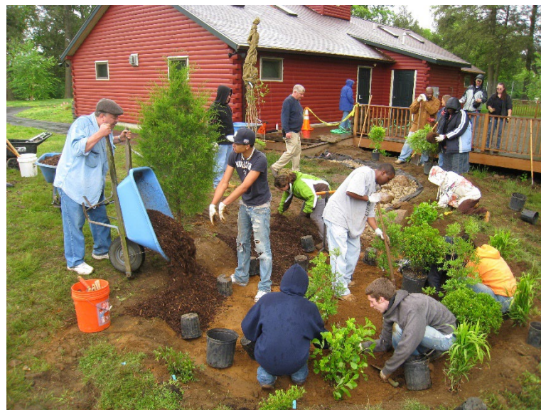
Many Sea Grant programs educate landscape professionals, municipal officials, homeowners, and students about the effectiveness of rain gardens as a way to limit the harmful effects of stormwater runoff. In this image, Volunteers help Connecticut Sea Grant build a raingarden in Bridgeport. Photo credit: Connecticut Sea Grant.
