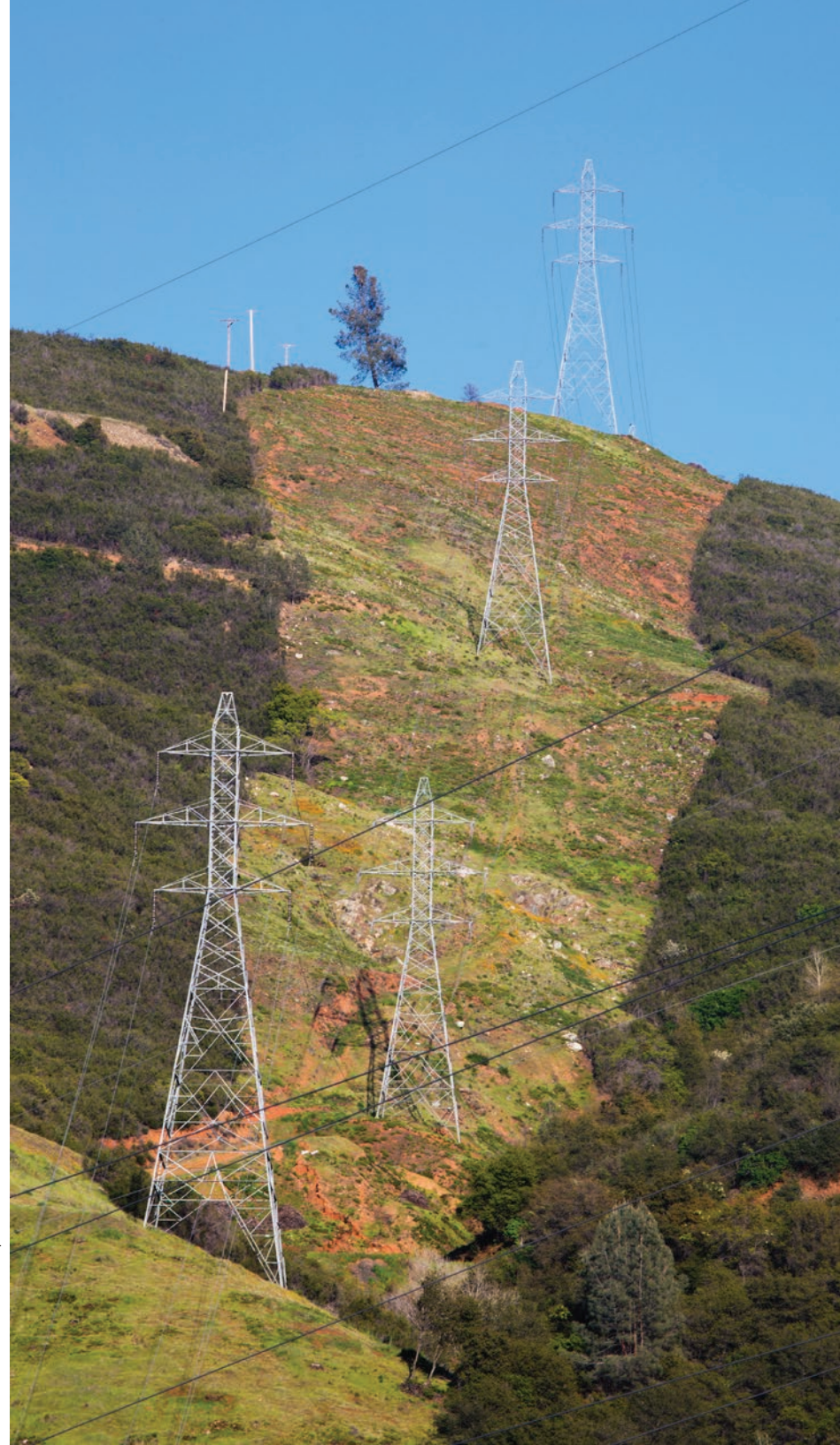
Transmission power lines in local watershed
