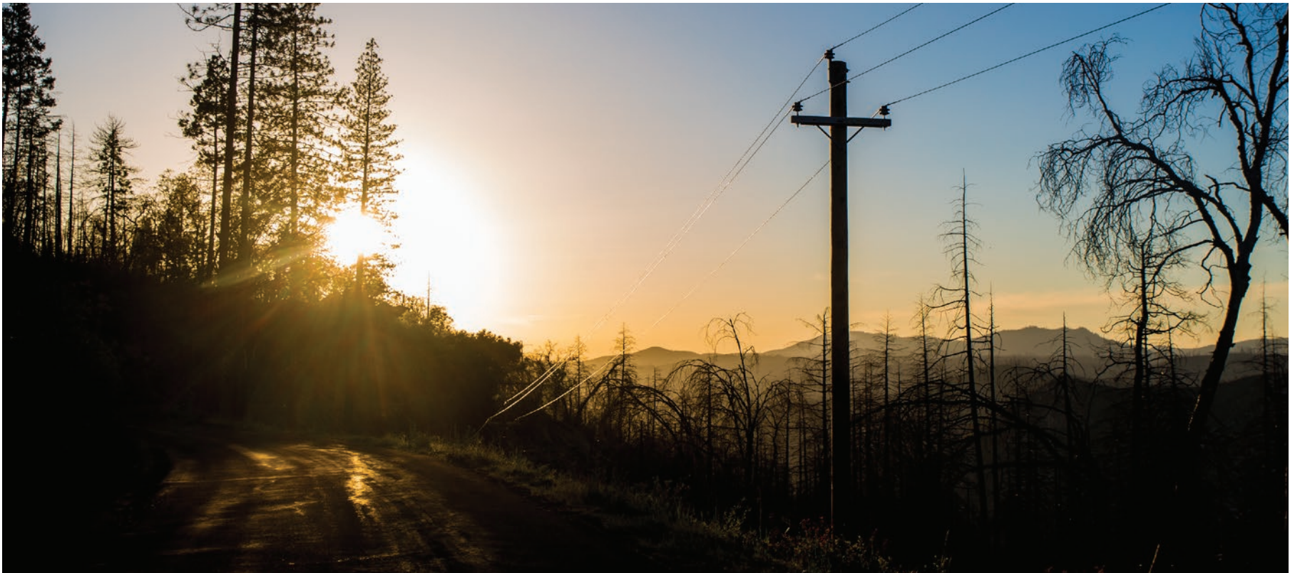
Local distribution power line near burn area
