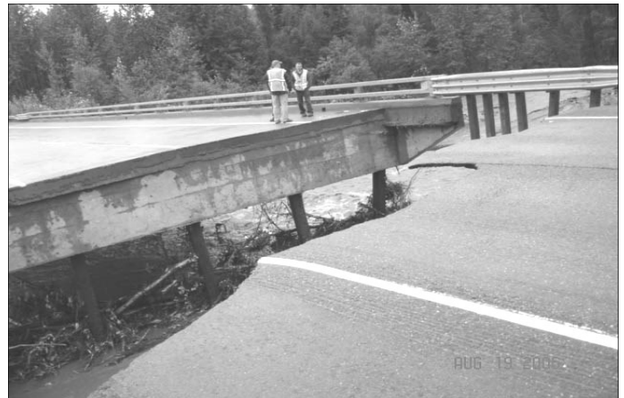
Washed out approach to bridge over Troublesome Creek on the Parks Hwy August 2006
