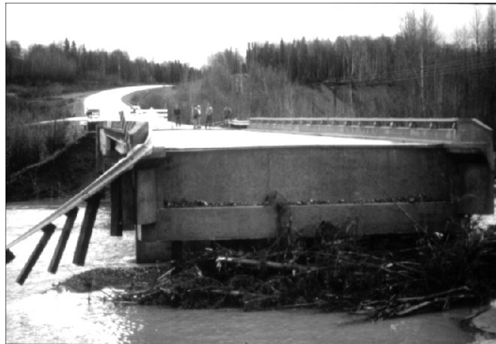
The approach to the bridge over Montana Creek on the Parks Highway washed out October 1986
