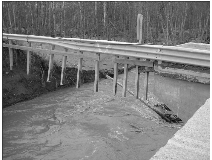
Bridge washed out over Deep Creek due to heavy rains October 2002
