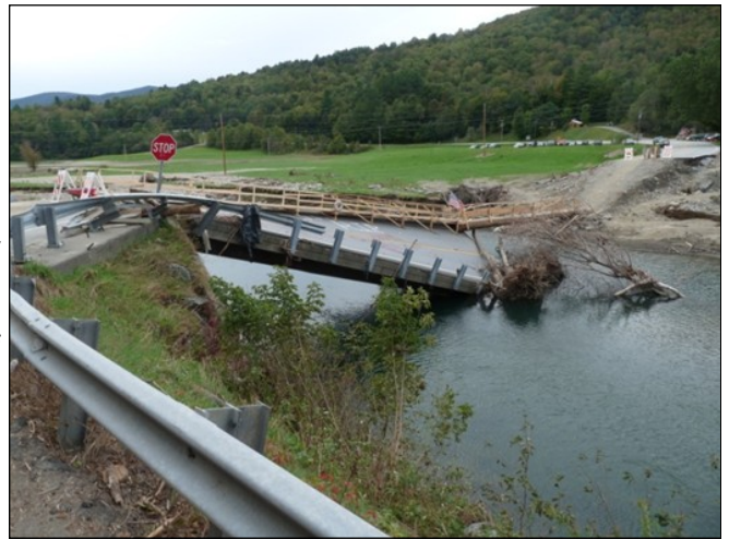
Bridge destroyed on Hwy 100 near Rochester, Vermont
