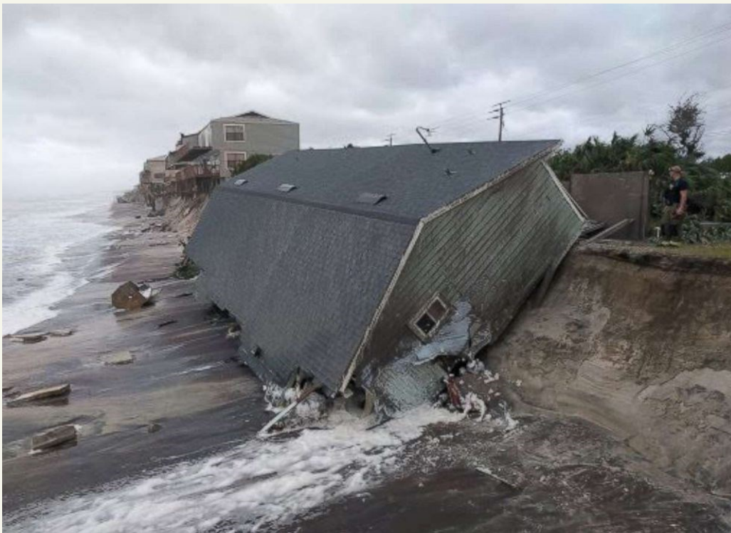
Damage from Hurricane Irma near Jacksonville, Florida. (Photo Courtesy ABC News)
