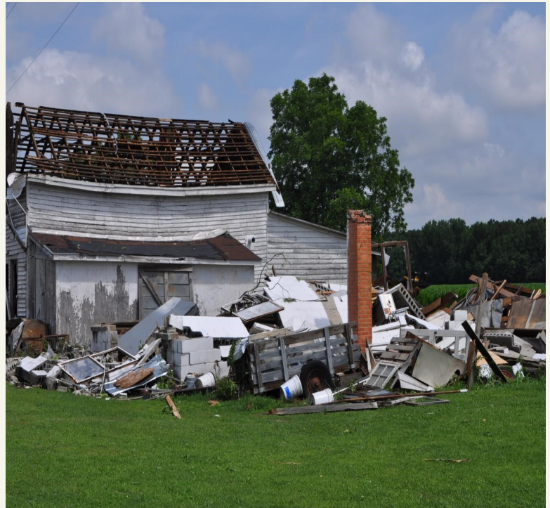
Damage near Bethel, NC (Photo by Caty Whitehurst)
