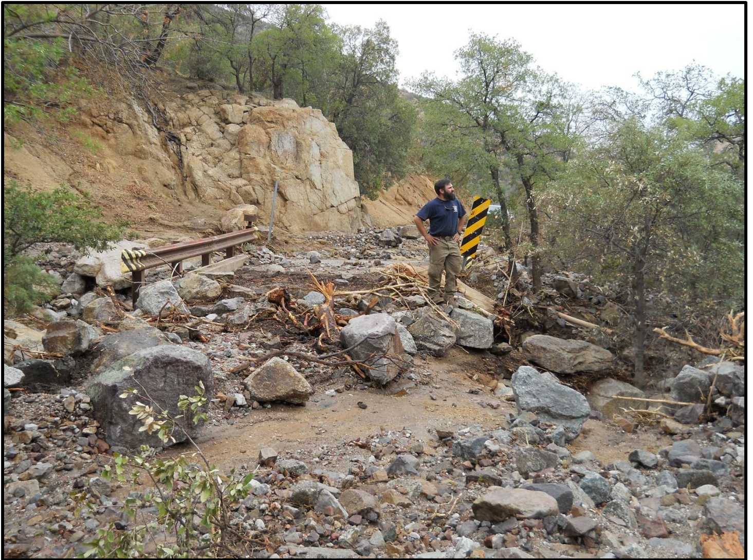
Figure 44. Bridge in Carr Canyon: bridge is approximately 0.2 mile upstream of the cross section (figure 39). This photo was provided courtesy of BAER team and was taken the day after the Carr Canyon flash flood.
