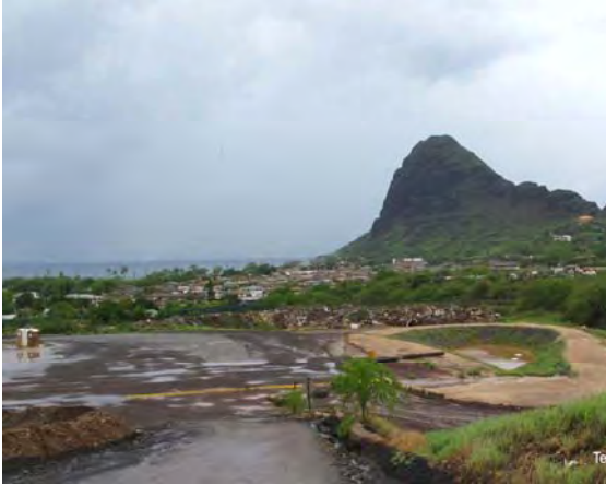
Newly install culvert and retention pond at the PVT Landfill in Nanakuli, Oahu, Hawai'i
