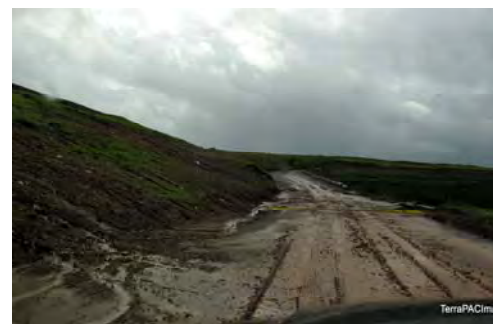
Road to landfill subject to erosion and washout that can cause closures during heavy rainfall
