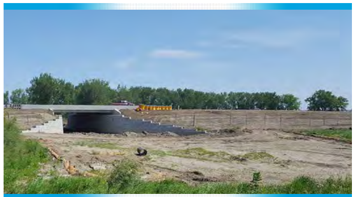
Lewis and Clark Bridge Wildlife Crossing
