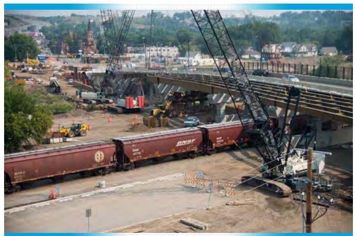
Construction and replacement of the US 83 Broadway Bridge over the Souris (Mouse) River and railroad tracks through downtown Minot
