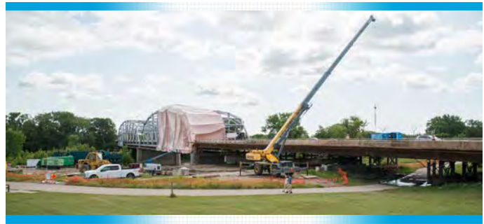
Kennedy Bridge project on US 2 over the Red River in Grand Forks District
