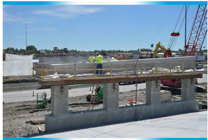
Construction on the Modified Single Point Intersection on the Sheyenne Interstate 94 Intersection Project in West Fargo
