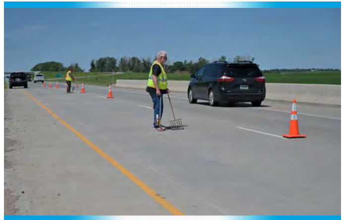
Fargo District employees look for delamination on a bridge deck using a process called chaining
