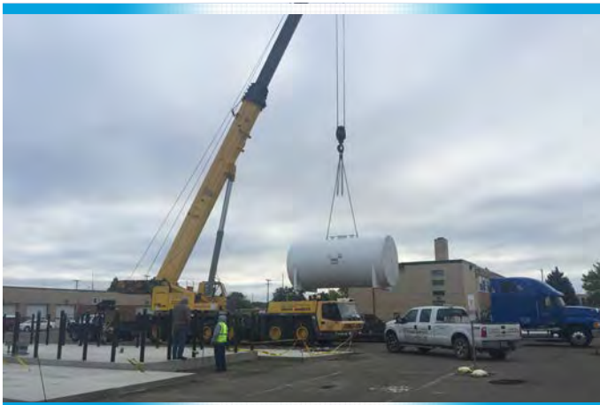
Large crane used to install new fuel tanks at the Bismarck District Shop
