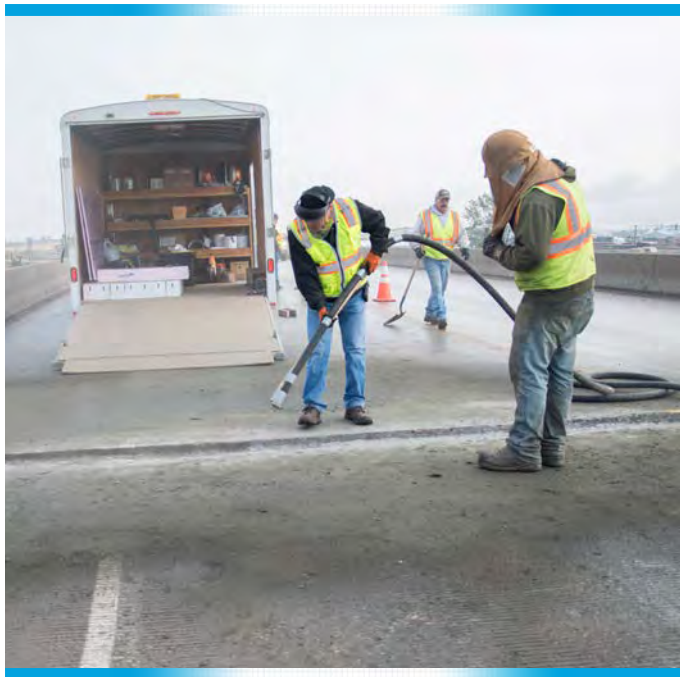
District employees learn a new maintenance process of joint repair on bridge on ND Highway 40 in Tioga
