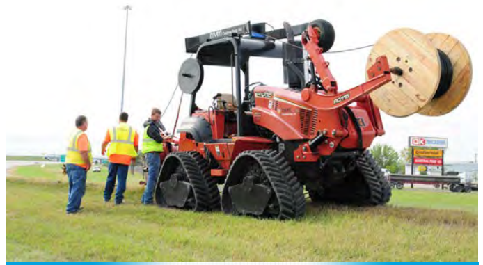
Fargo District installed fiber optic cable under and alongside the roadway for traffic counting and monitoring speeds
