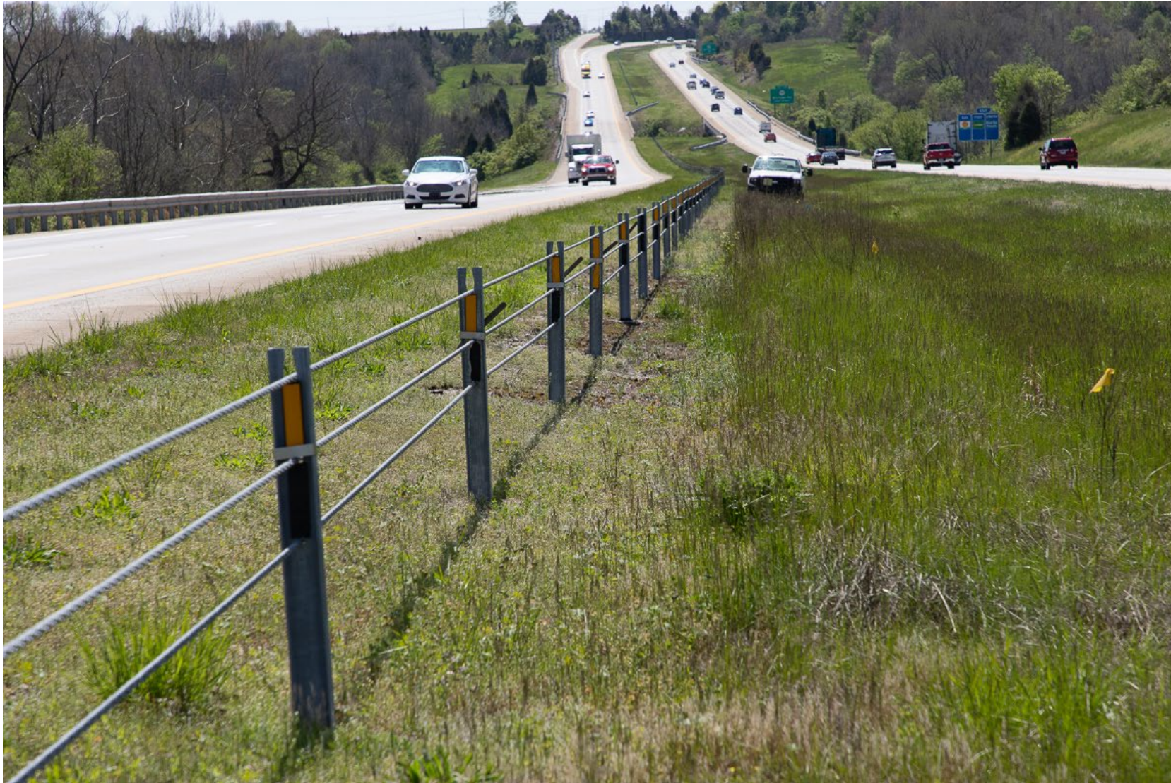
Figure 2: View of Plots in the Cable Barrier Trial on April 27, 2020 (342 Days After Treatment) Visual effects of the treatments at the beginning of the next season.
