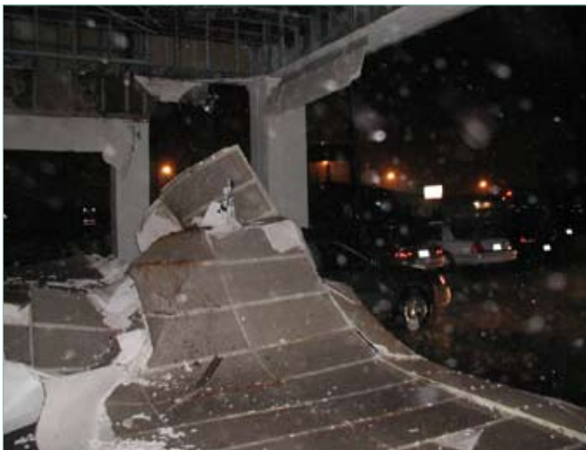
Figure 3: Collapsed sheetrock on Greg Postel's car in Mississippi (note the anemometer protruding through the sheetrock on top of his car).
