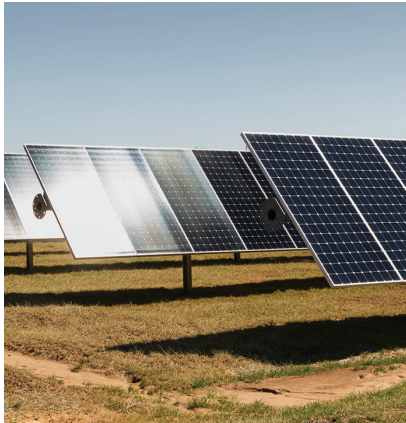
Our Maiden, North Carolina data center is powered by our biogas fuel cells and three solar arrays.
