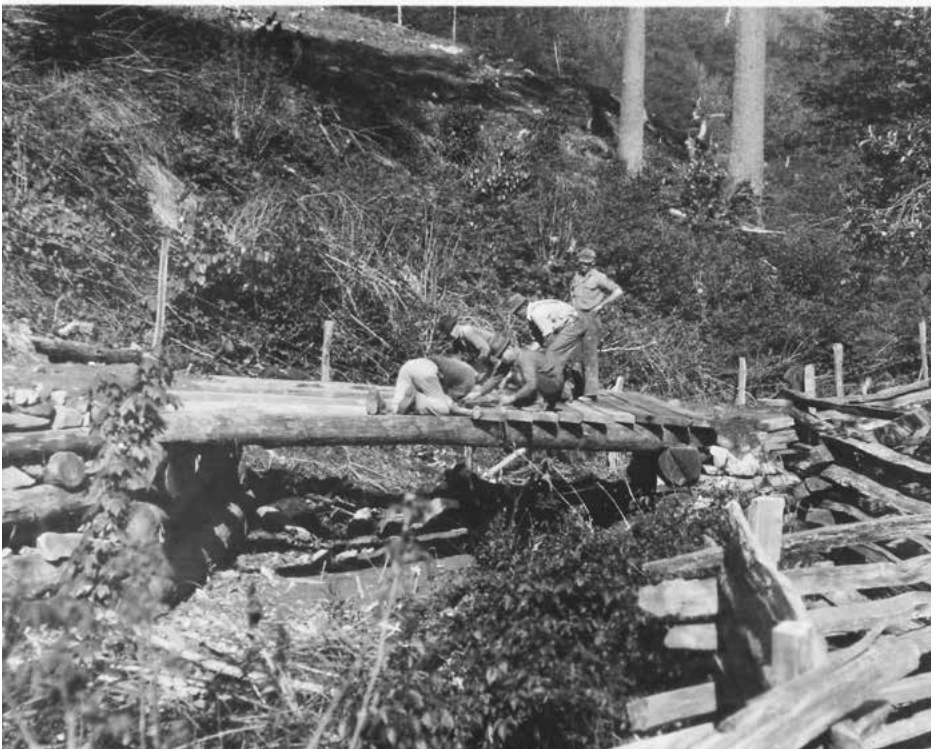
Eastern Band of Cherokees work at flooring the connecting link between the Lower Bunches Creek section and Upper Bigwitch in the Wrights Creek section.
