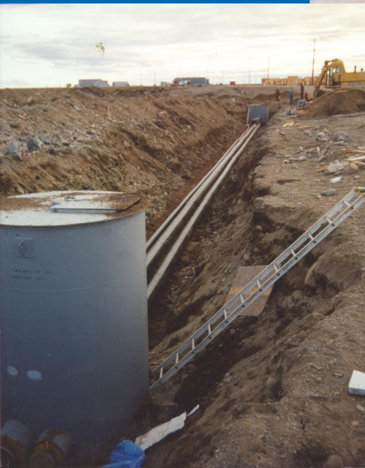
Piped water and sewer in Rankin Inlet NU
