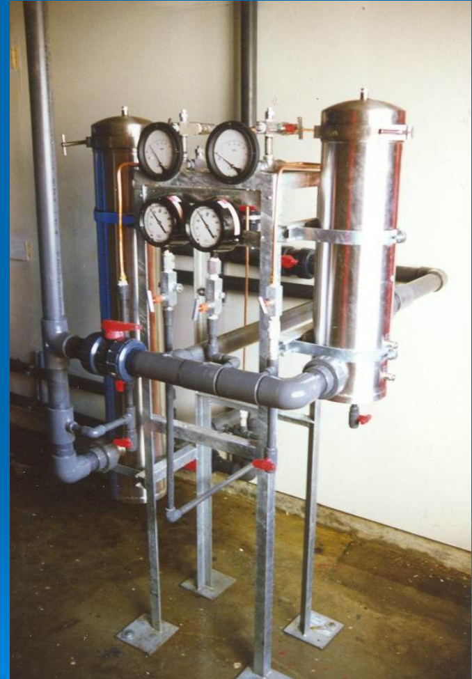
Cartridge filtration system in Carcross YT
