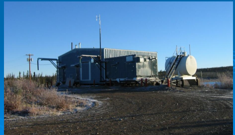
Water treatment facility Tsiigehtchic, NT
