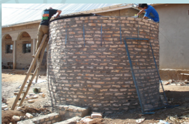
Univ Minnesota - Engineers Without Borders Rainwater Harvesting System, Uganda
