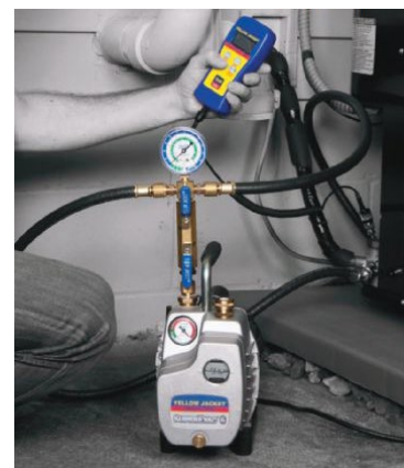
Figure 8.6. Vacuum pump used in this workshop configured for its primary use in refrigeration-circuit cleaning.
