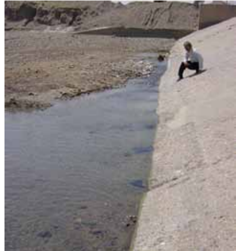
Figure 3: Water emerging from weepholes
