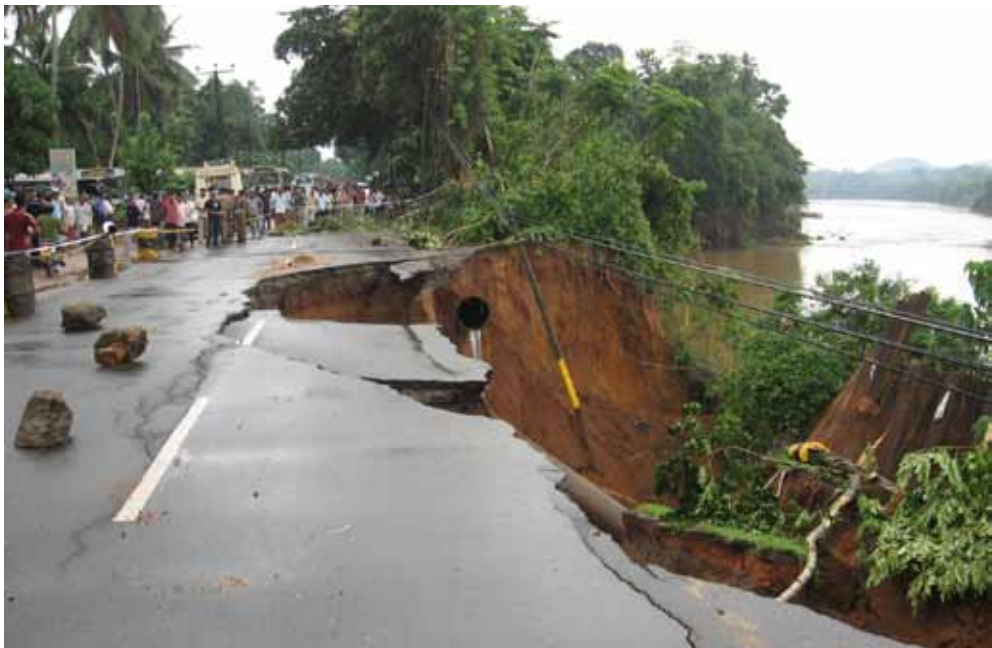
Figure 1: Kelani river bank erosion due to sand mining. A domestic water supply pipe line underneath the road got damaged and city water supply got disturbed for several days. (Photo: Badra Kamaladasa, Irrigation Department of Sri Lanka)
