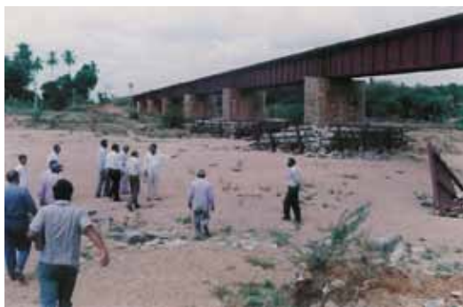
Figure 3: Railway bridge foundation frequently being repaired due to sand mining across Uttara Pinakini river in Gauribidanur taluk, Karnataka, 2002. (Hemalatha, A.C. et al. 2005)
