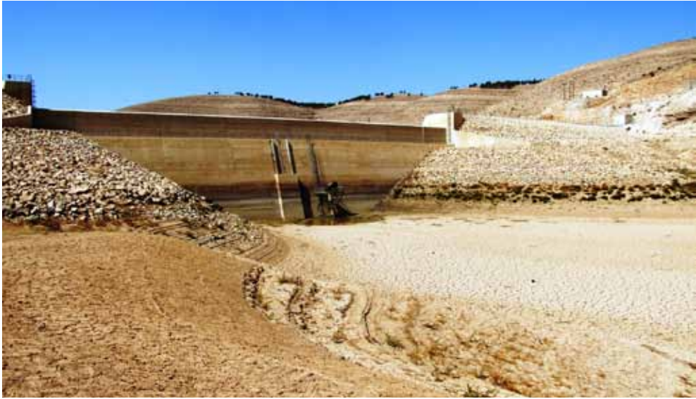
Figure 3: Sediment Accumulation at the Bottom of the Wadi Wala dam has led to the Closure of the Bottom Outlet and the lower Draw-off Pipe
