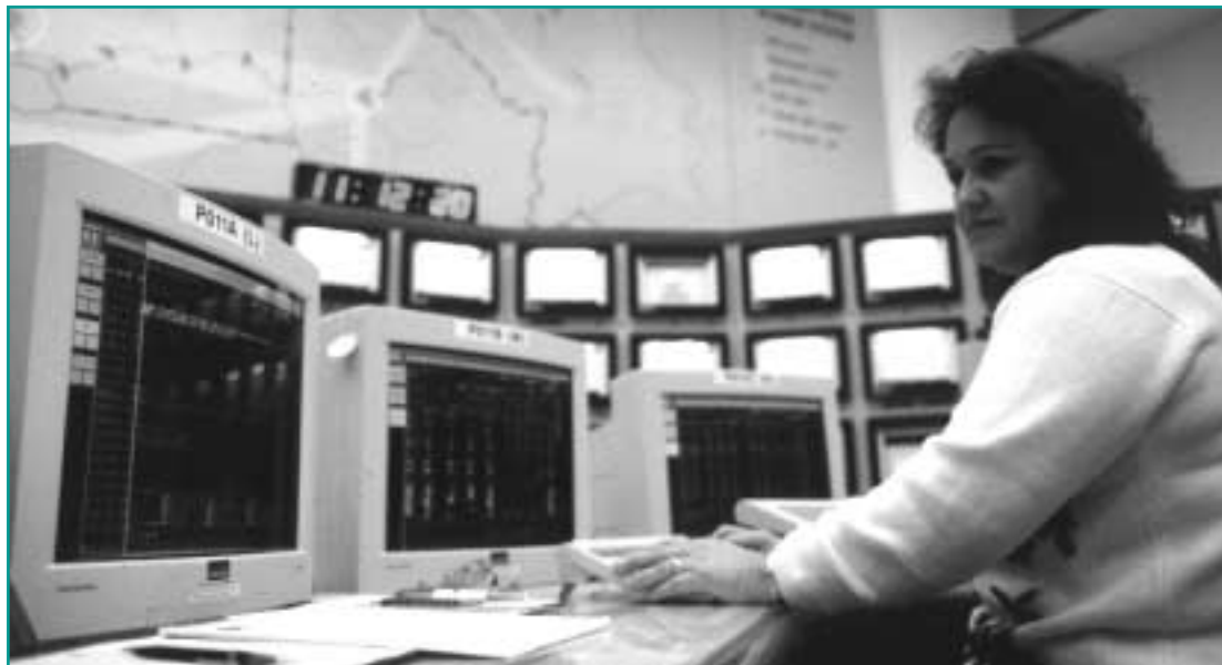
Operators work around the clock to meet load with the best combination of resources.
