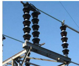
230 kV Disconnect Support
