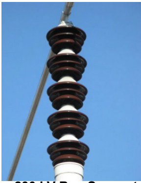
230 kV Bus Support
