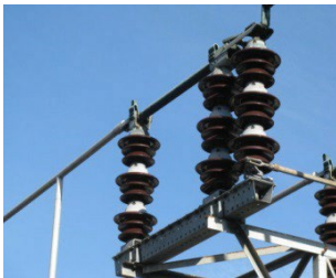
115 kV Disconnect Support
