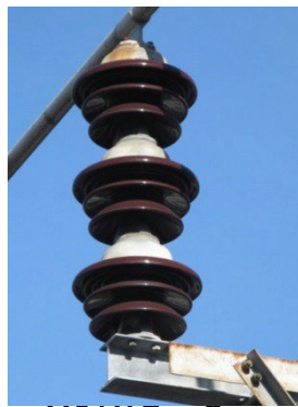
115 kV Bus Support
