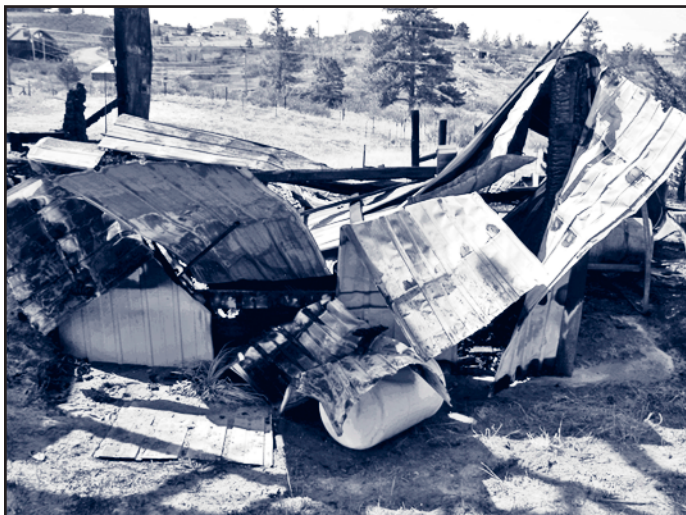
FIGURE. Shed debris resulting from home-based biodiesel production fire — Colorado, 2006
