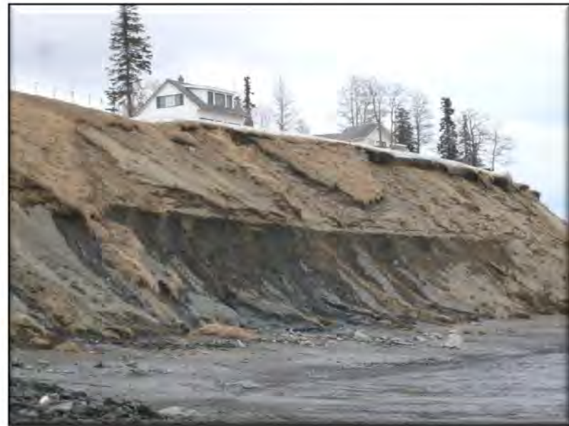
Bluff Erosion along Kenai River
