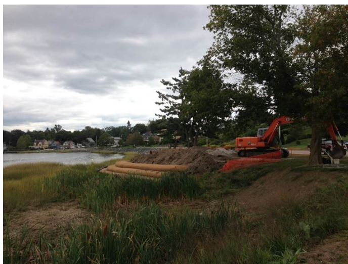
Stillhouse Cove, Cranston had a severely eroded bank which was a safety hazard. The bank was reshaped to a gentler slope to reduce wave energy and lessen erosion. Sand-filled coir logs were added to the bank and native grasses planted. (Photo: CRMC, Save The Bay)
