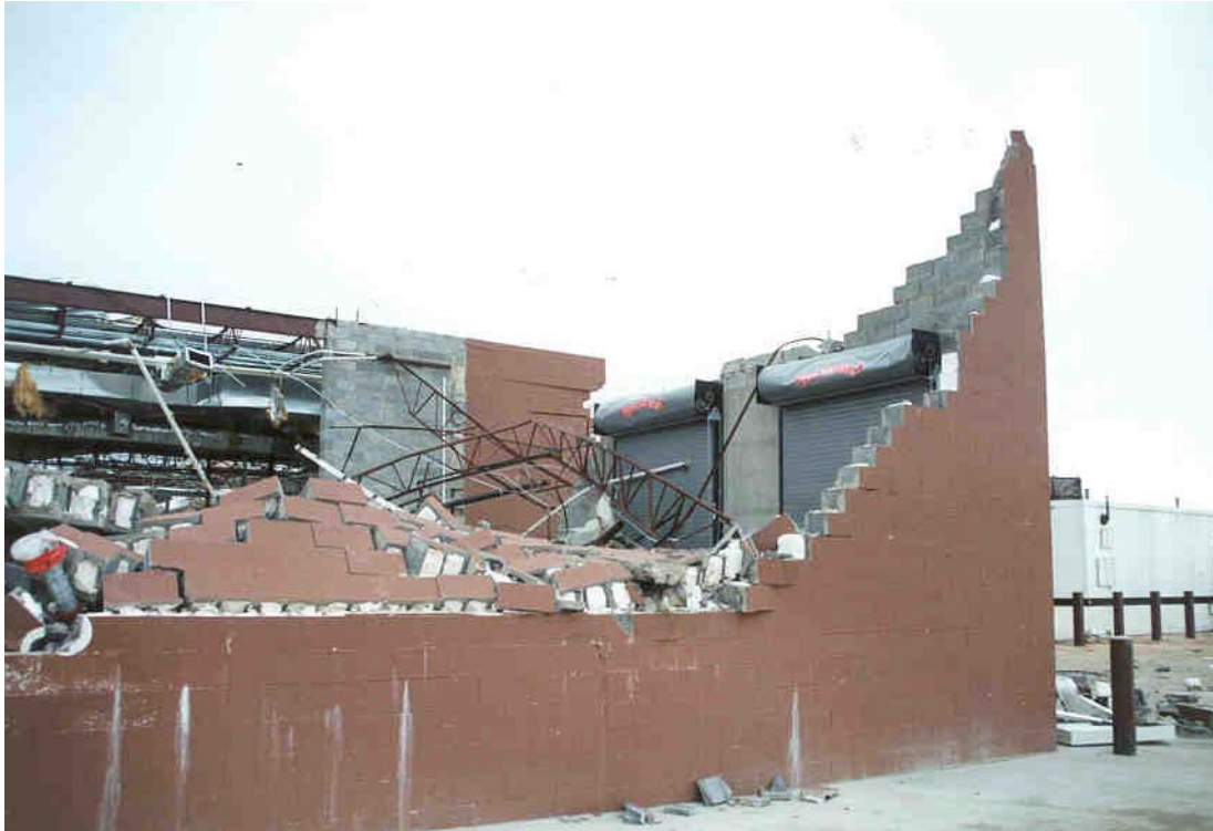
Figure 6. Englewood Village Market Place, internal pressurization
