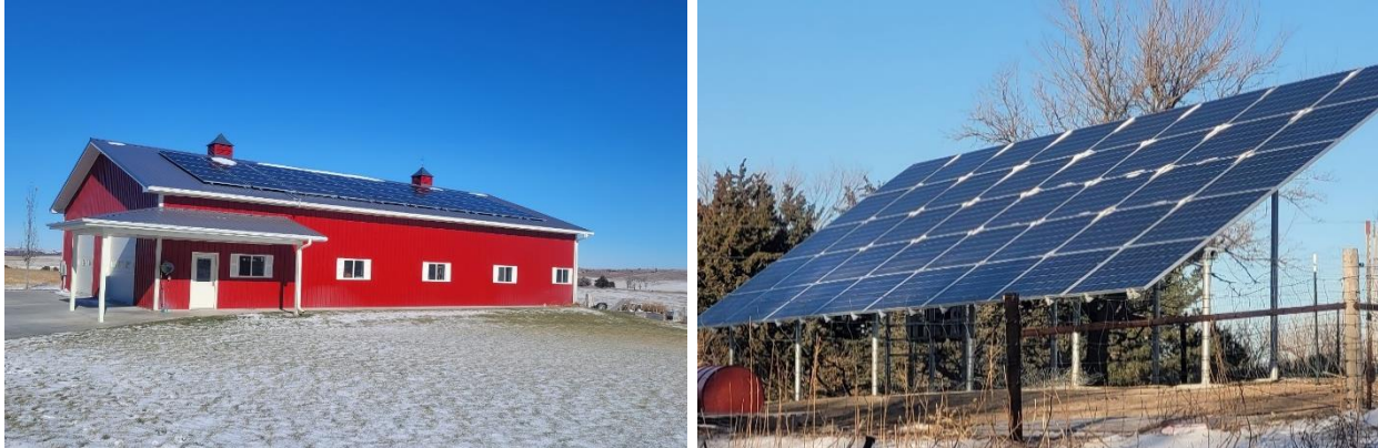
Top: Roof-mounted 22.8 kW solar array, Broken Bow (2022); Bottom: Ground-mounted 15.6 kW solar array, Scotia (2022).
