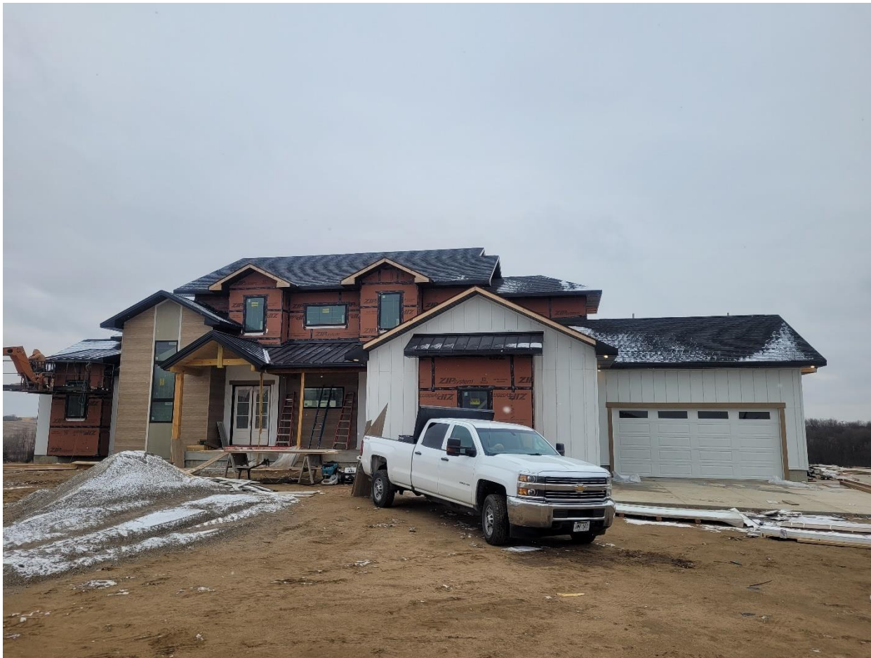
Construction of a new above-code, energy-efficient, single-family residence was completed with funds from the Dollar and Energy Saving Loan's Energy Efficient Housing Program, Firth (2022).
